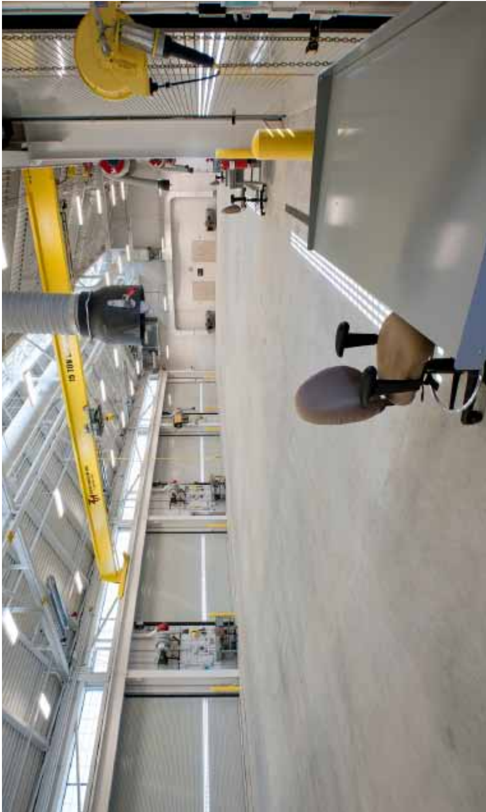
Inside the Vehicle Maintenance Facility, two massive cranes - 15-tons and 12.5 tons respectively - extend the width of the building.
