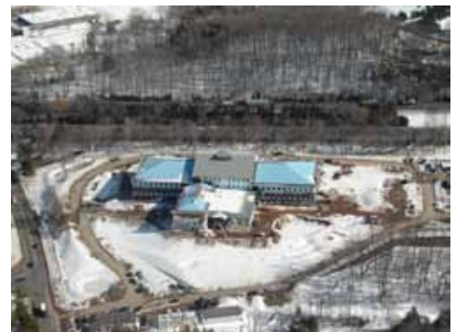
The exceptional snowfalls of the 2010-2011 winter posed yet another challenge to the fast-tracked project schedule.
