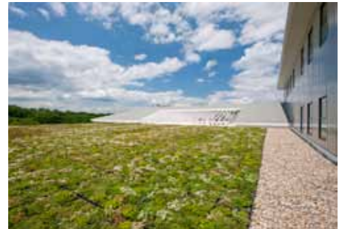
The 10,000 sf green roof on the Training Center is the first in the nation-wide Reserve Center program.
