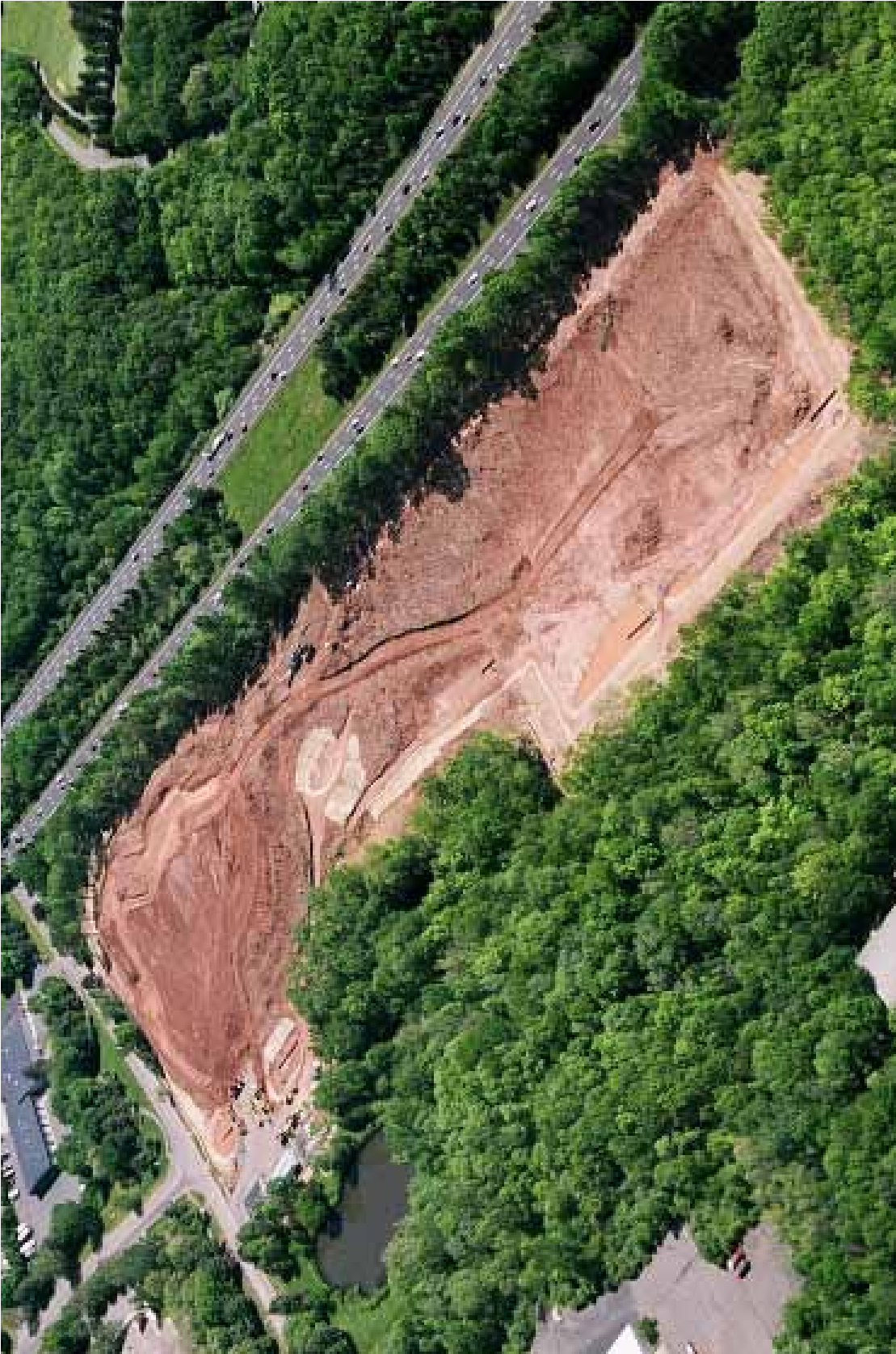
The 42-acre site adjacent to Interstate 91 included steep slopes and wetlands. The massive sitework effort included the removal of more than 500,000 cy of earthwork and the construction of 1880 lf of 25+ foot high retaining walls along the wetlands. At the height of construction, trucks hauling materials were leaving the site every two minutes.
