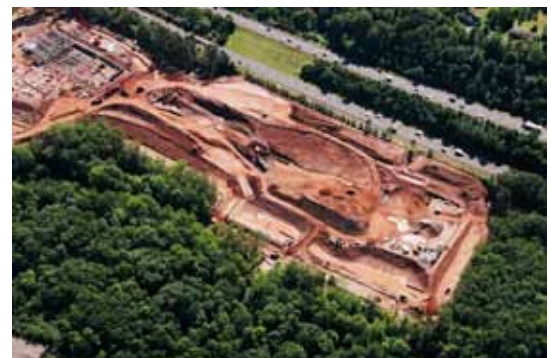
The massive sitework component of the project called for the removal of 500,000+ cy of soils, with dramatic grade changes.
